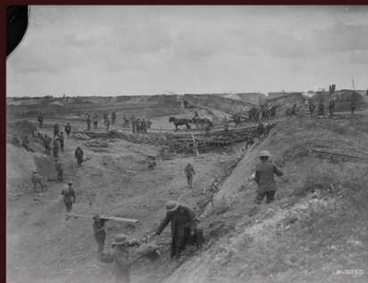
The famous Canal du Nord showing construction and cutting across which Canadians crossed with their supports and supplies. Advance East of Arras. Library and Archives Canada MIKAN 3329287
